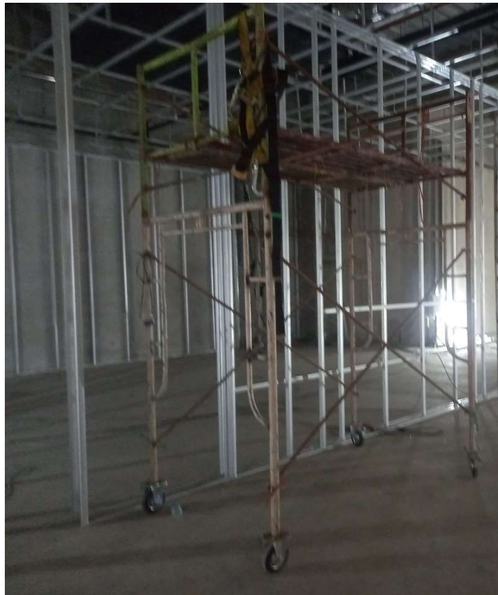
Photo 08. Perancah Frame Bergerak Dengan Handrail & Roda Terkunci Saat Bekerja. Mobile Frame Scaffolding with Handrail & Locked Wheel in Work Progress.
