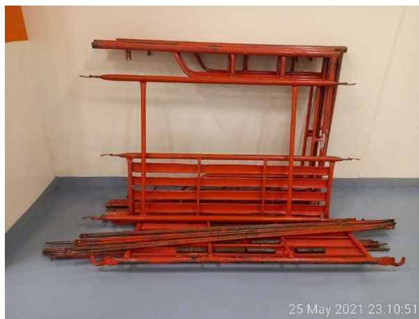
Photo 10. Scaffolder Mempersiapkan Besi Perancah Frame Sebelum Dirakit untuk Bidang Kerja Kuat & Stabil. Scaffold Technical Prepare Iron Frame Scaffolding Before Installed To Be Strong & Stable Platform.
